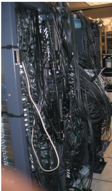
Traditional Cluster Cabling
